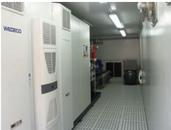
Containerized ozone system type SMO
