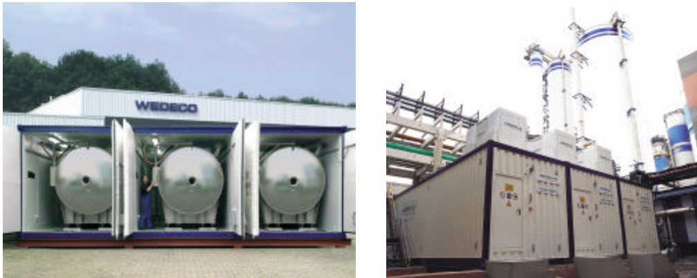
Figure 4 – Ozone containers from WEDECO installed at the VCP Jacarei mill.
